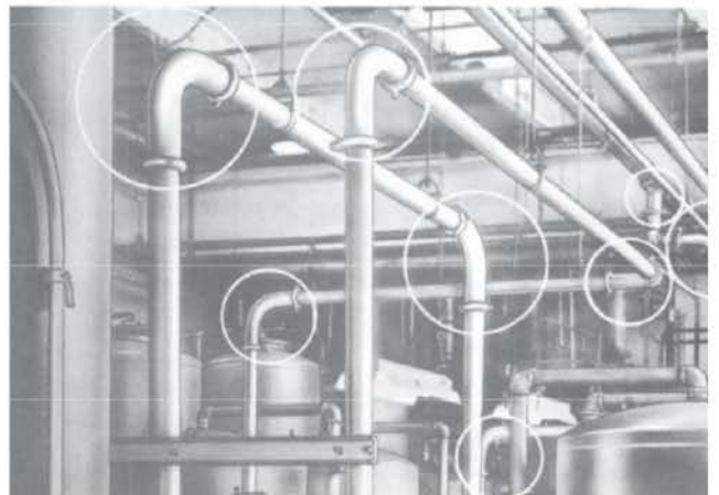
A large dry-cleaning plant uses Flexmaster joints to connect piping at elbow junctures.
