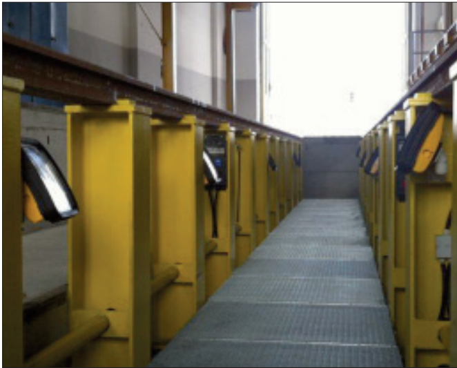
Prima Light – working pit
