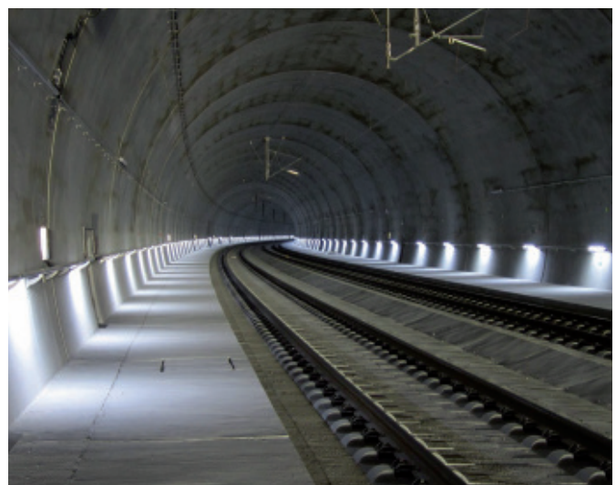
AmbitLED - handrail lighting, railway tunnel
