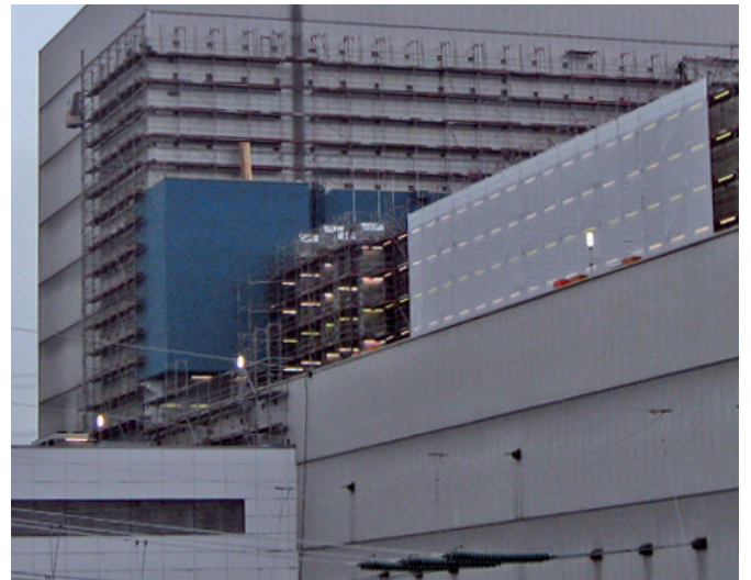
APOLLOLED - scaffolding illumination on an industrial building
