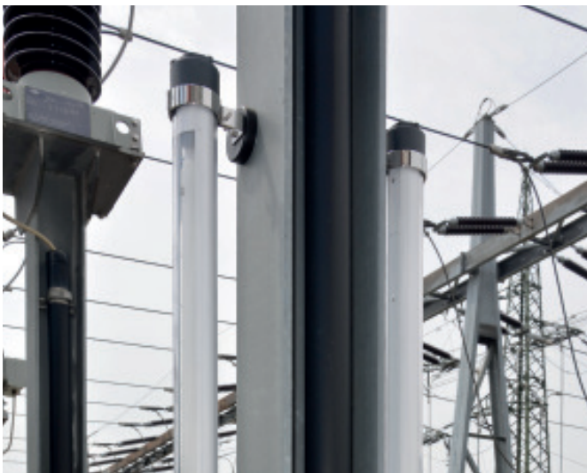
StreamLight 70 – transformer station
